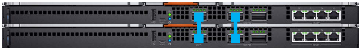
Figure 9 MX5108n SmartFabric VLTi cabling
